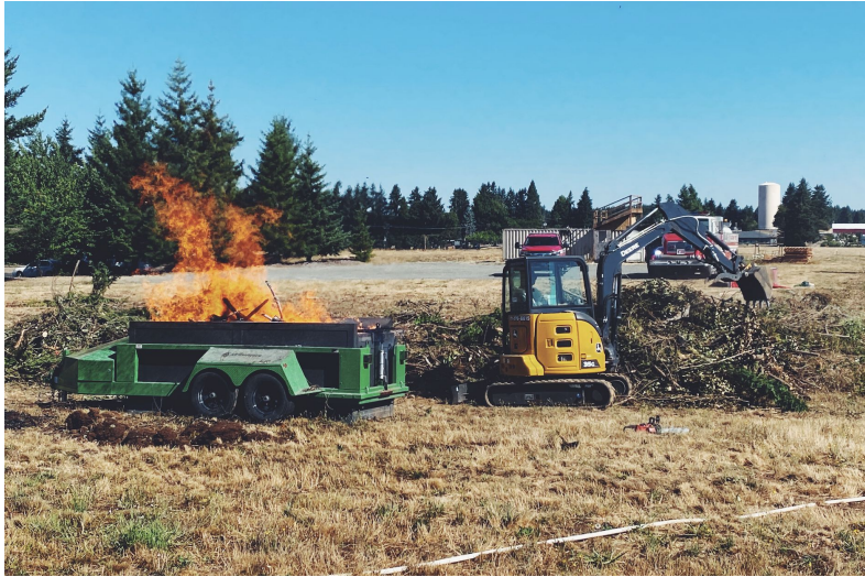
Air Curtain Incinerator
