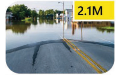
SCDOT Hurricane Helene, 2024
