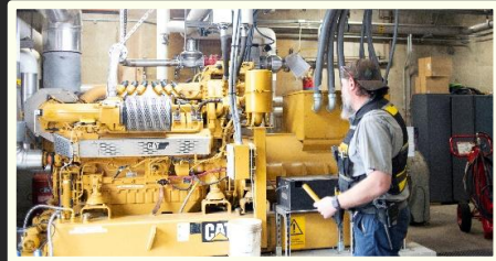
2023 – Biogas cogeneration engine at Tri-City WRRF
