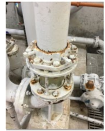
Picture 11. Primary Pump Station Piping General
