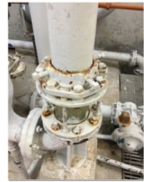
Picture 11. Primary Pump Station Piping General
