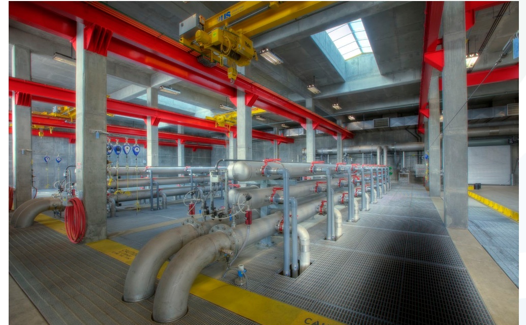
Membrane Bioreactor (MBR) (2011)
